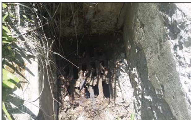
Figure 36 Drop inlet, WCSWCD
