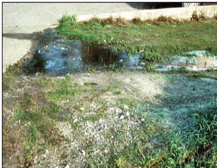
Figure 30 Surface septic failure Image courtesy of EPA and King County, WA
