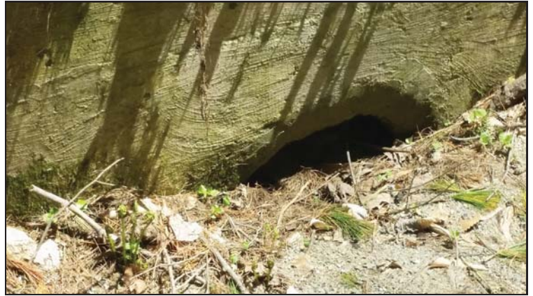
Figure 31 Culvert that is full of sediment and debris, WCSWCD
