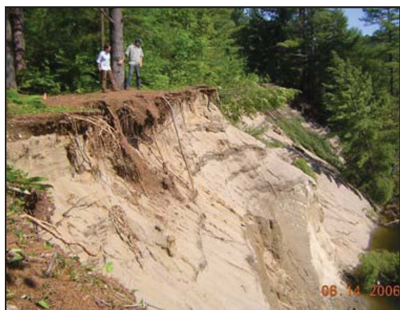
Figure 19 Example of steep, sandy streambank on Schroon River, WCSWCD
